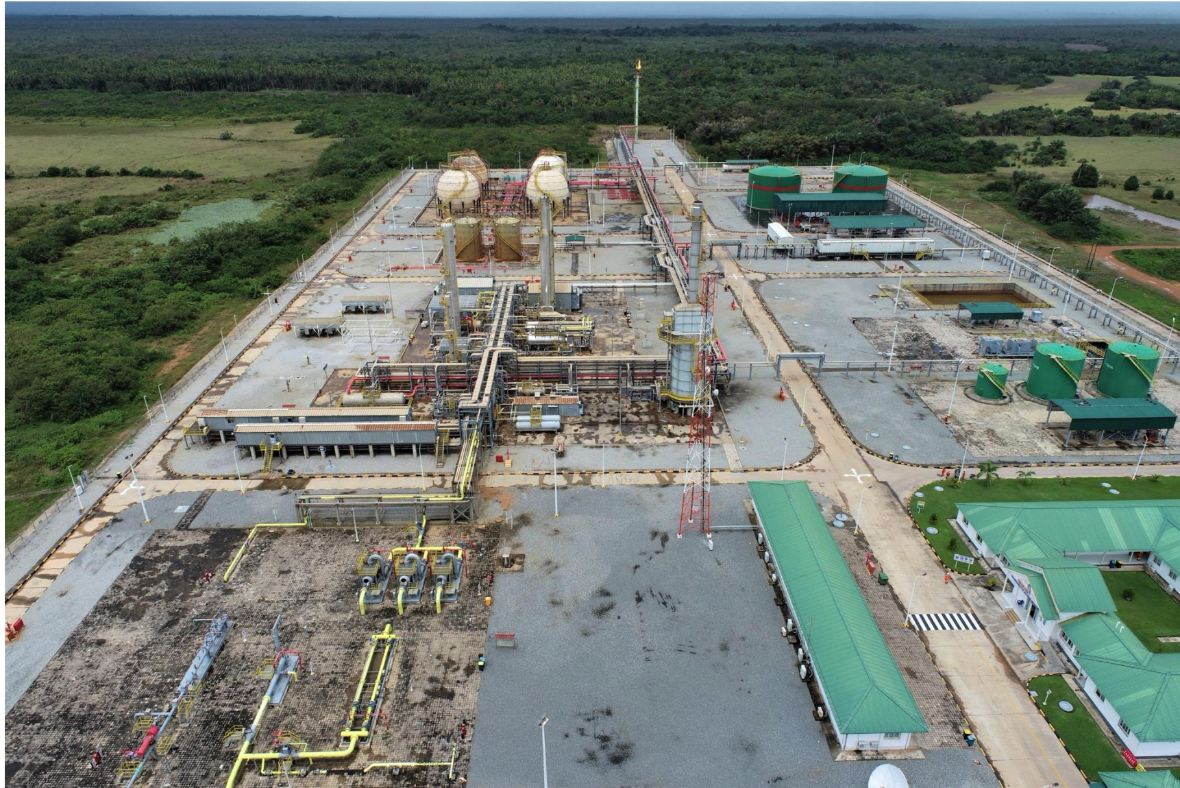
Figure 1 Gas Processing Plant Train 1
